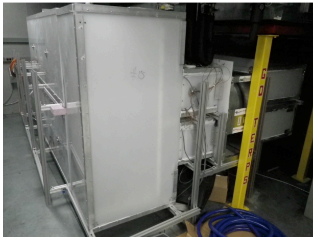
Figure 8. Ducts connected together.
