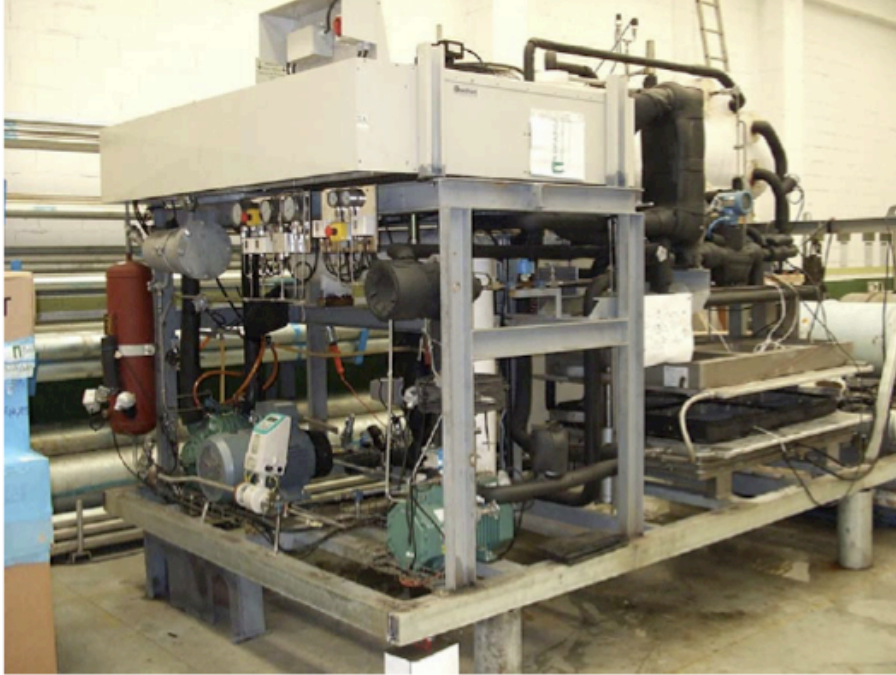
Figure 1. Photograph of the experimental prototype of the cascade refrigeration system with CO 2 and NH 3 refrigerant [1].
